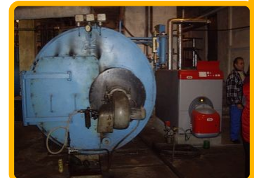
The old and new boilers
